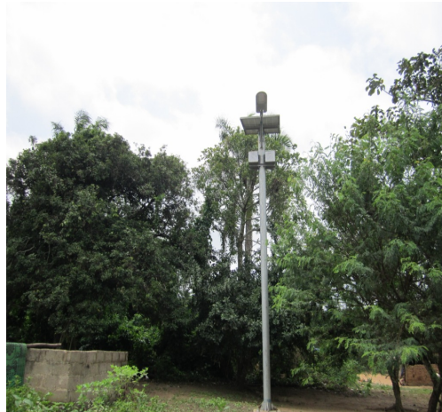
Plate 12: Oponda Community Solar lighting system - functional
