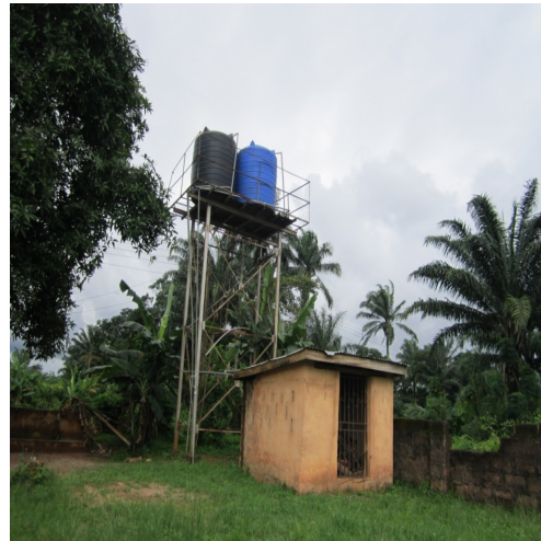
Plate 4: Non-functional community water supply project
