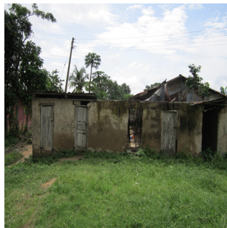
Plate 6: Apostolic Primary School, Ugom, Latrine – Out of use
