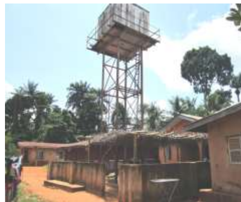
Plate 2: Okonkpon water supply scheme (Non-functional)
