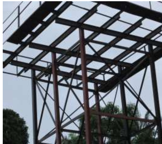
Plate 16: Kalai Ibiama uncompleted water supply project
